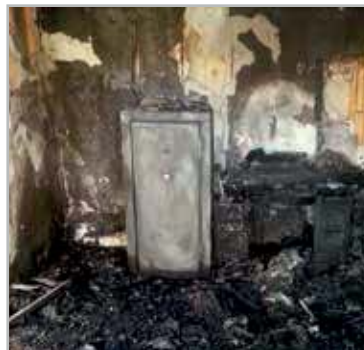
William's fire started 2 feet from his safe. The fire burned for about 45 minutes.
